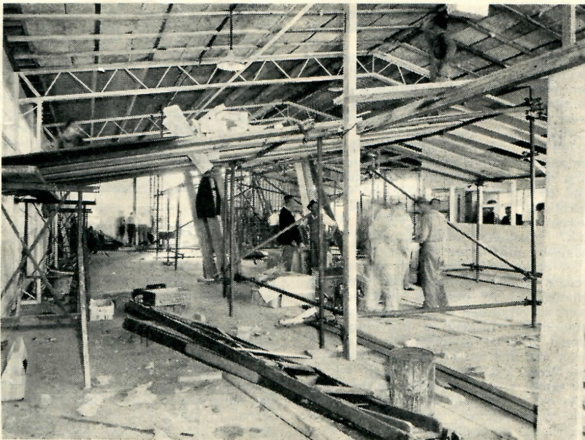
Fig. 6.—Scene inside the Line Depot Building on the Day of the Fire. New M.D.F. is being Erected and Roof Insulation is in Progress.
