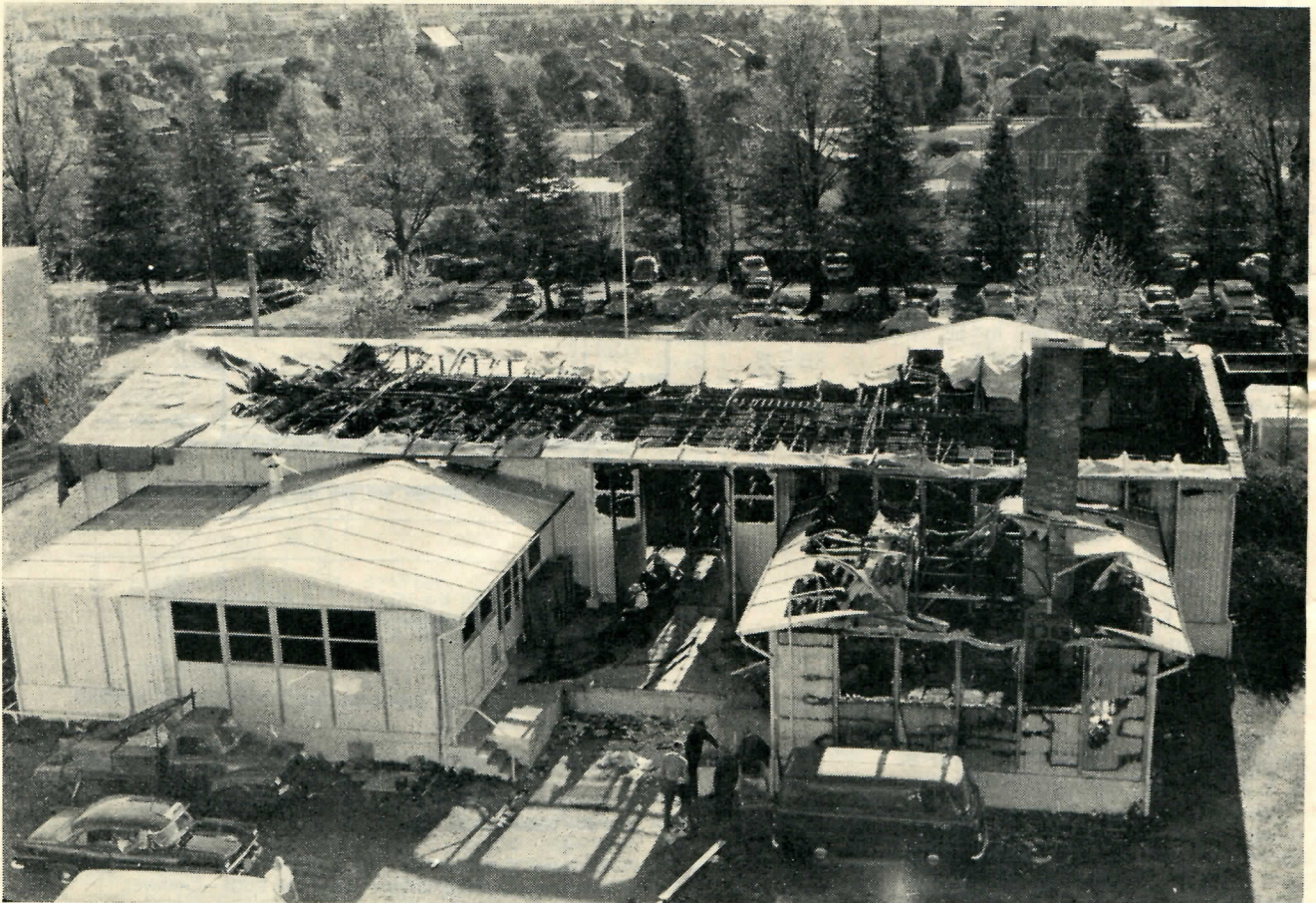
Fig. 1.—Looking down on Damaged Building, showing Destruction of Air Treatment and Equipment Areas.
